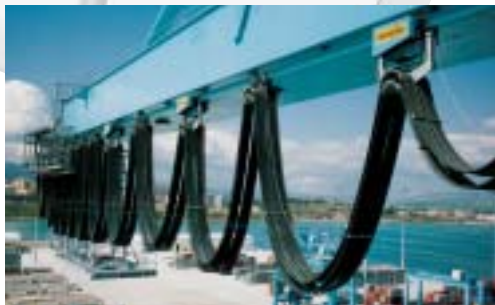
Offshore container crane with motorized cable trolley system
