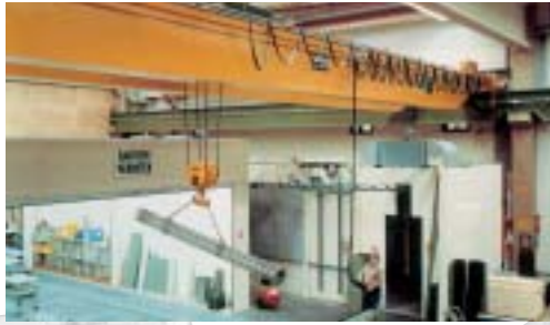
Current supply system with ideal control unit trolley on a bridge crane
