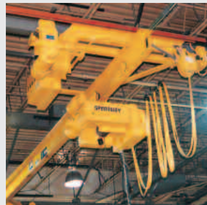
Louden crane with Speedway hoist.
